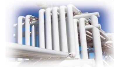
Industrial Gases Pipeline
